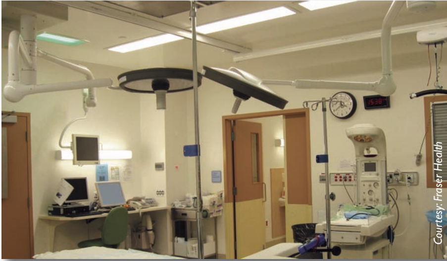
OR with the Ceiling Lift System.
